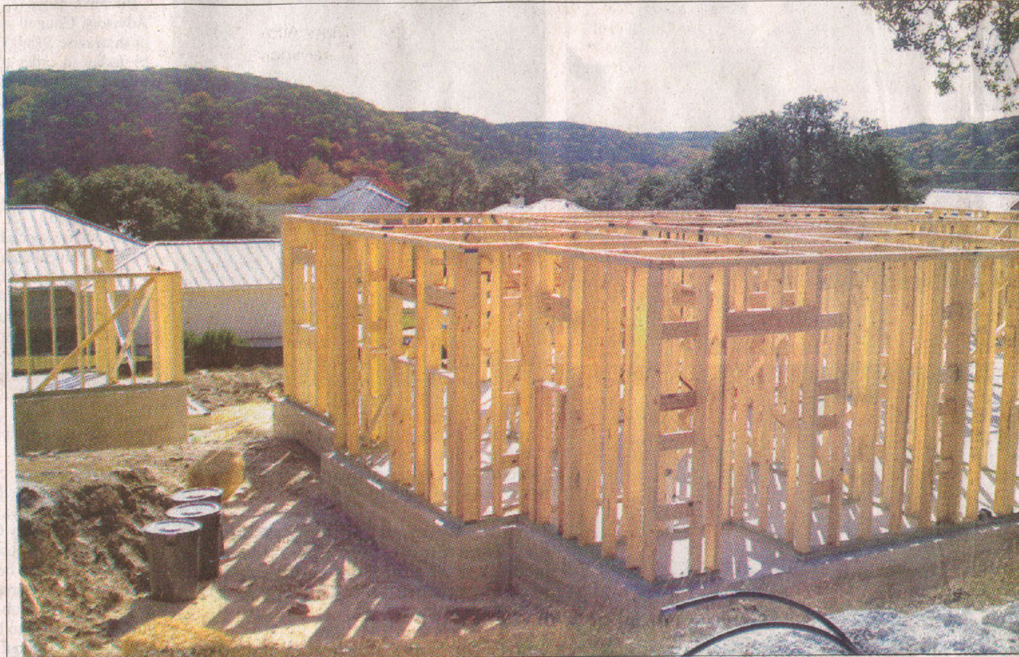
The green house being built by Griz and Karen Adams is in its early stages of framing. Note in the foreground the coil hoses sticking out of the ground. They tie into the geothermal system the Adams family is employing to maximize heating and cooling efficiency.
